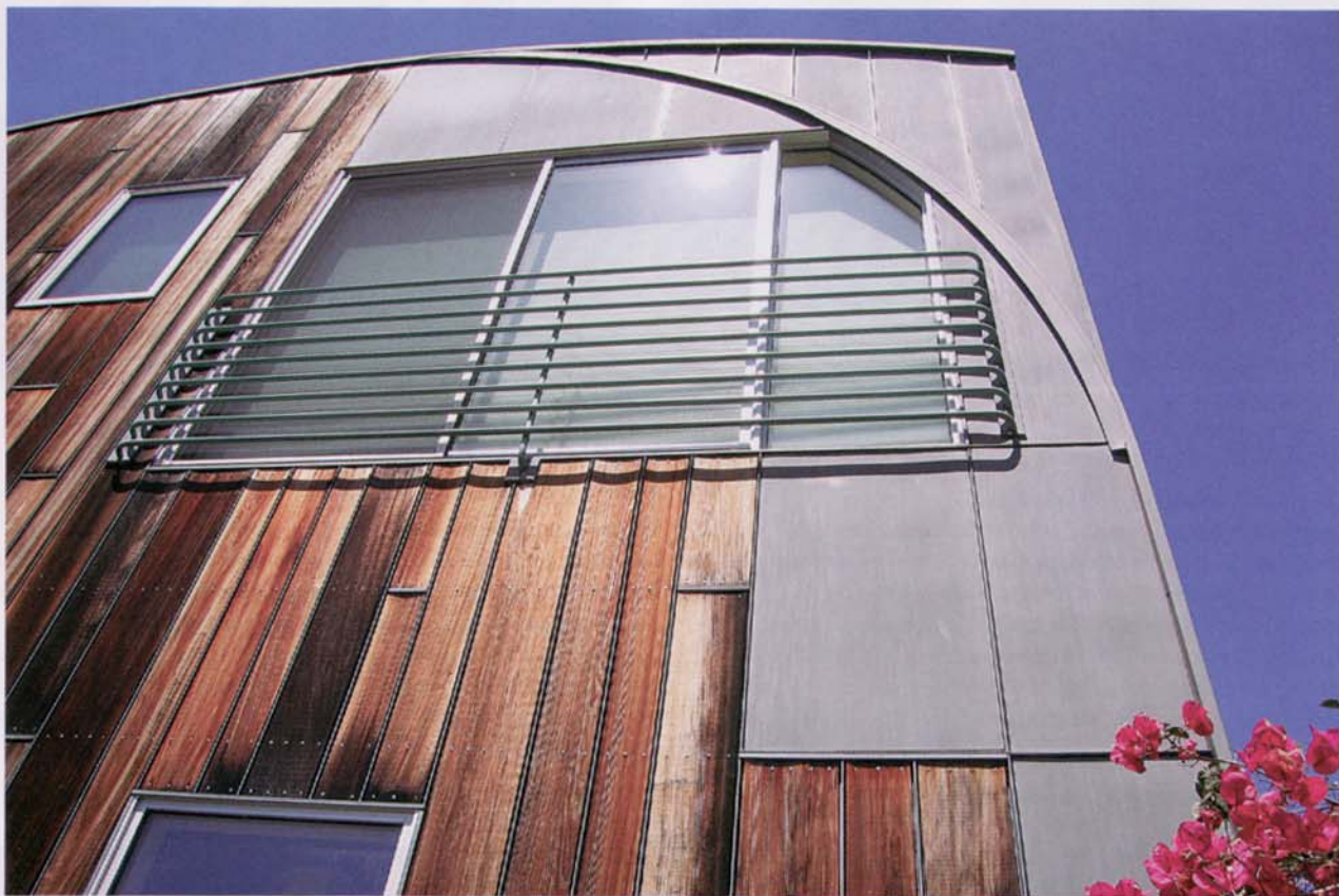
The exterior is clad in redwood from old Northern California wine vats and zinc sheeting.
